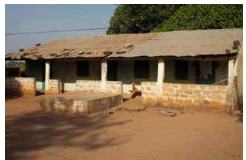
Sololo Staff accommodation block - inside is worse!
